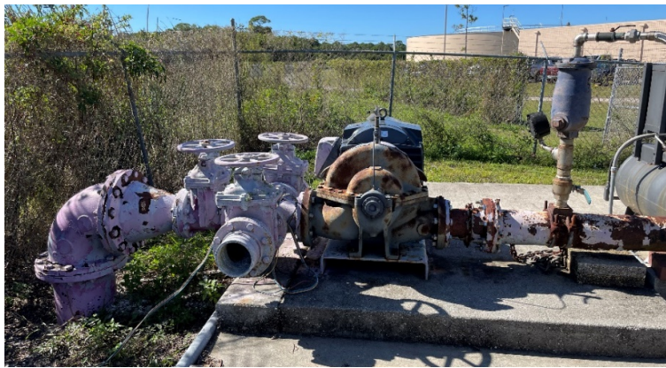
5-6. Western pump is scorched; pipe corrosion.
