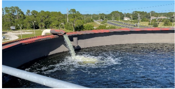
2. Corrosion around the top of the reuse storage tank.
