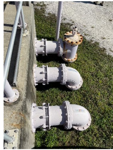
4. Bolt corrosion on pump station overflow pipe.
