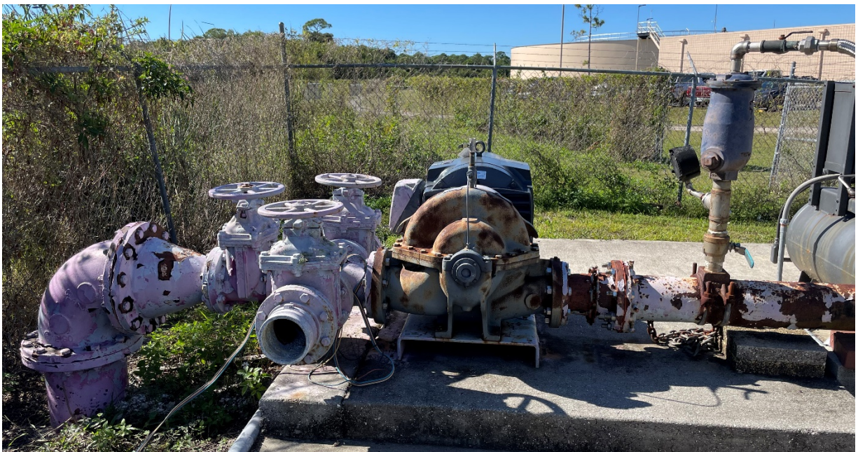
Figure 11: Western Irrigation Pump
