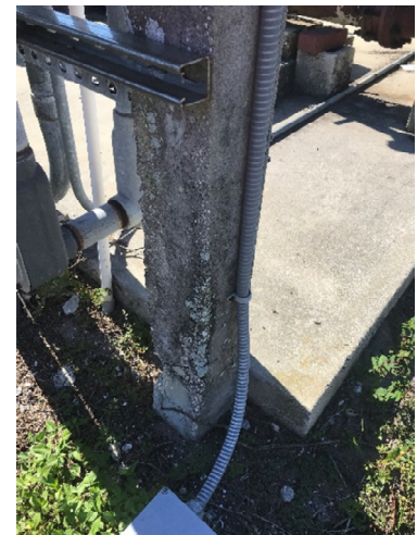
7. Electrical support pole concrete is crumbling.
