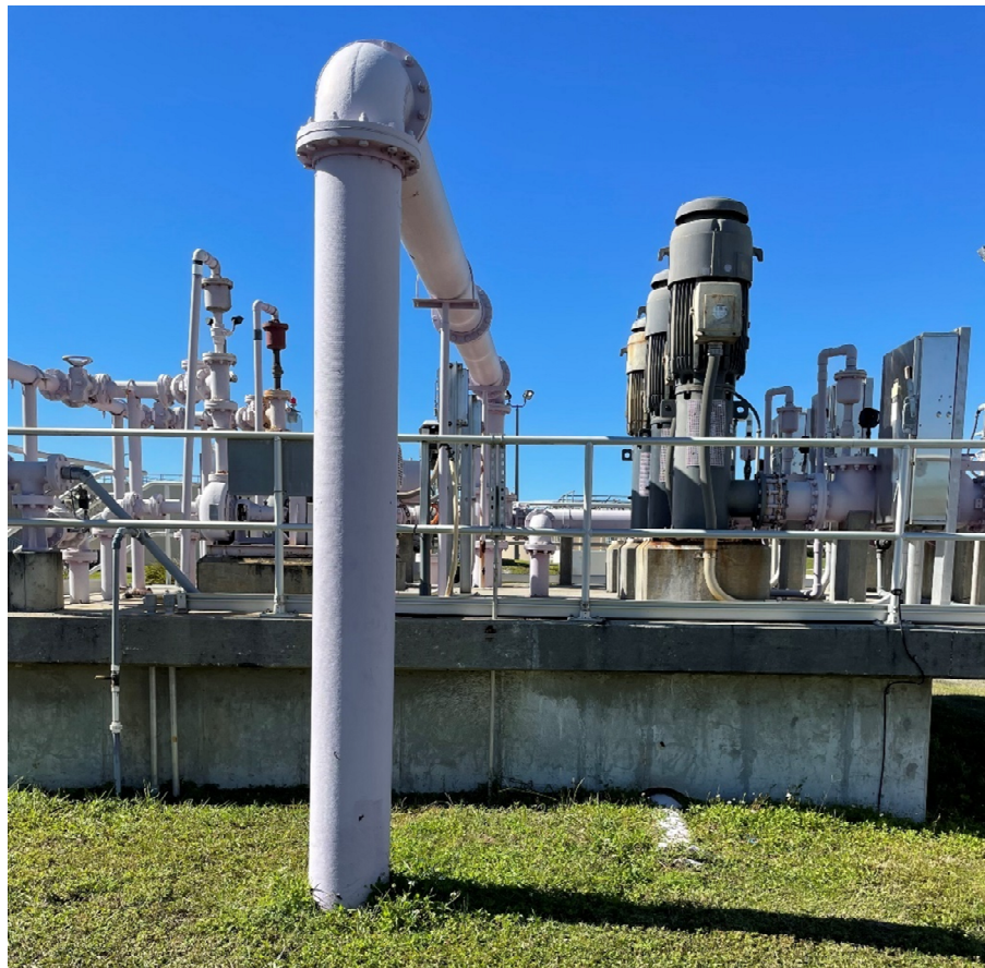
Figure 8: Reuse Storage Tank Influent Pipe
