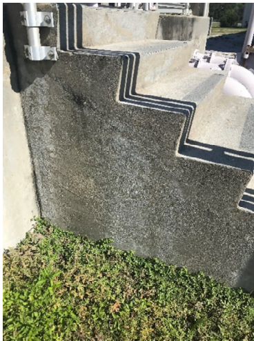
5. Crack in steps up to effluent pump station.
