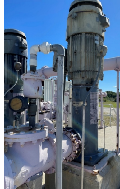
Figure 7: Effluent Pump at South WRF
