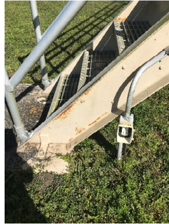
5. Corrosion on and underneath stairs up to the reuse storage tank.
