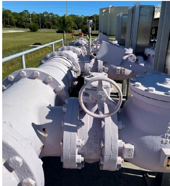
Figure 6: Effluent Pump Station
