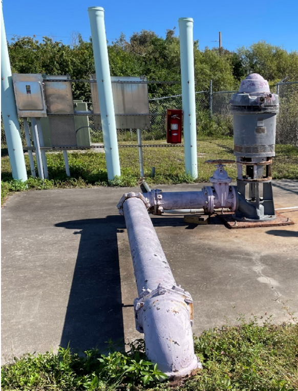
Figure 12: Eastern Irrigation Pump
