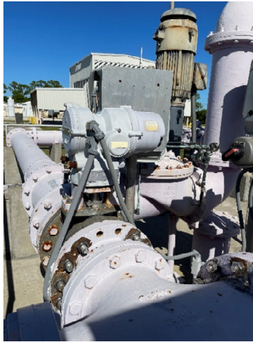
3. Flow meter piping and bolts to ASR Well are uncoated and corroding.
