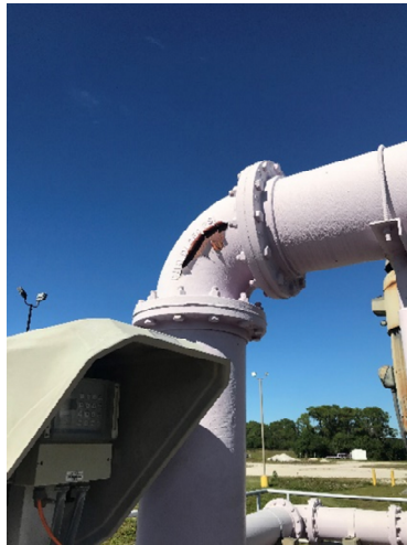
6. Pipe corrosion at the effluent pump station.
