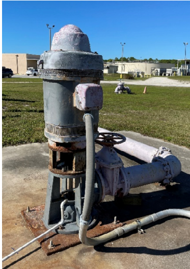
3. Eastern irrigation pump and base plate are corroded.
