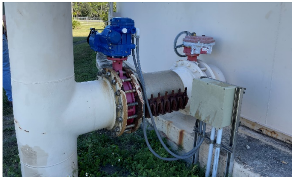
3-4. Corrosion around the bolts on the Flowserve Valve; Top of manual valve is weathered.
