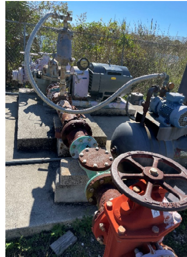
4. Western irrigation pump piping is uncoated and corroded.
