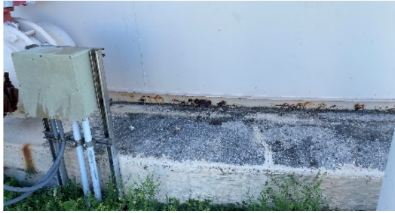
1. Corrosion around the bottom of the reuse storage tank.
