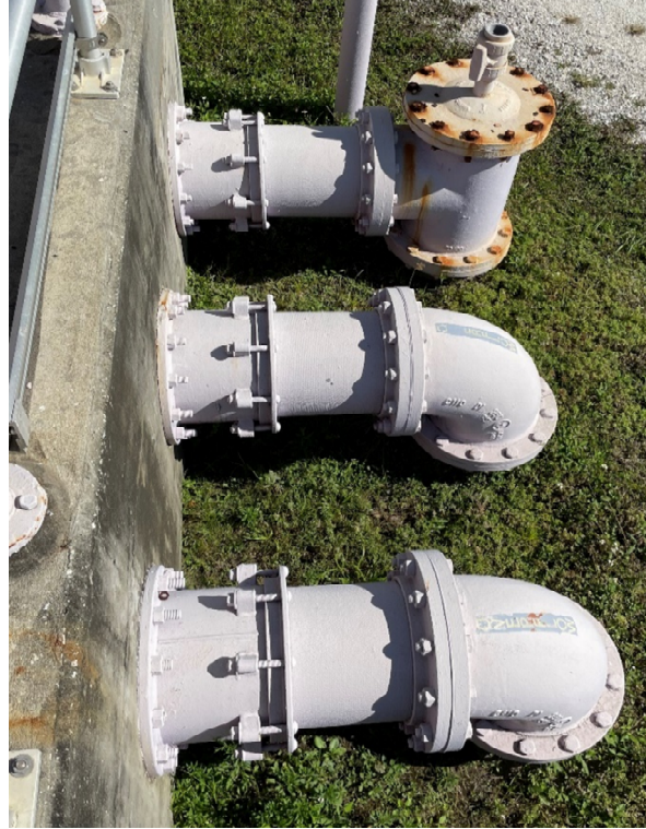
Figure 13: Overflow Pipes to Irrigation Pond
