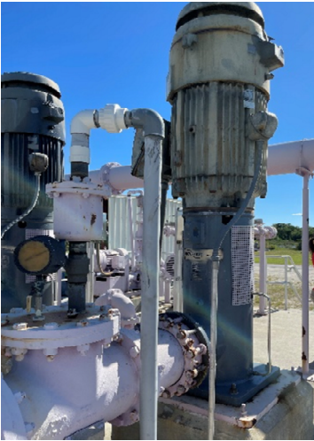
1-2. Corrosion around uncoated bolts; pump base plates are corroding.
