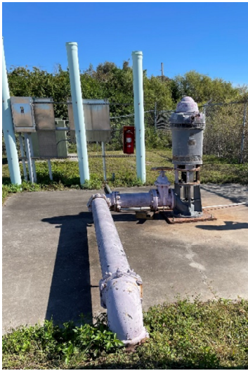
1-2. Crack in concrete pad at eastern irrigation pump; minor pipe corrosion.
